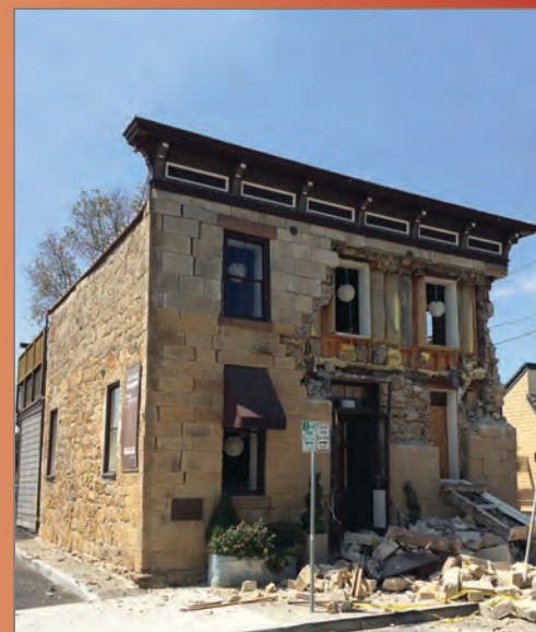
Damaged building in downtown Napa. Photograph by Erol Kalkan, U.S. Geological Survey.
