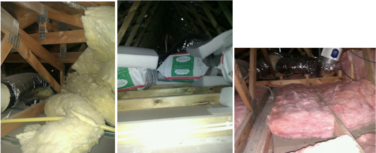
Figure 12 Examples of ceiling insulation rated as poor
