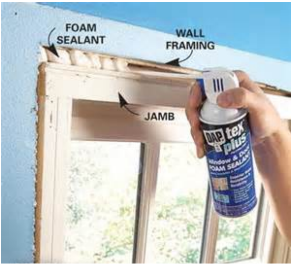
Figure 25 Expanding foam sealant used to fill gap between window and house frame
