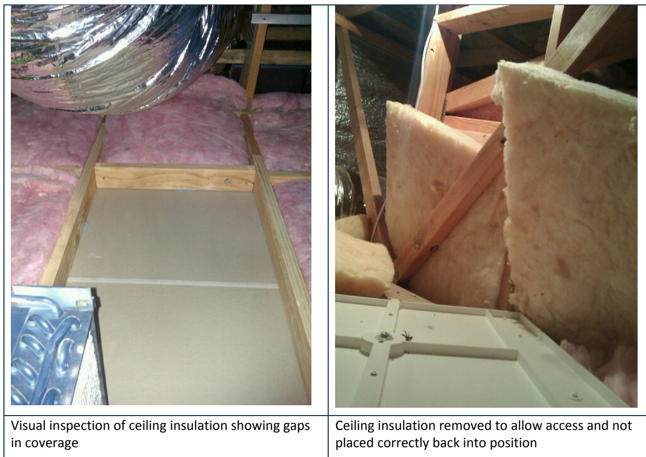
Figure 5 Examples of poorly installed ceiling insulation
