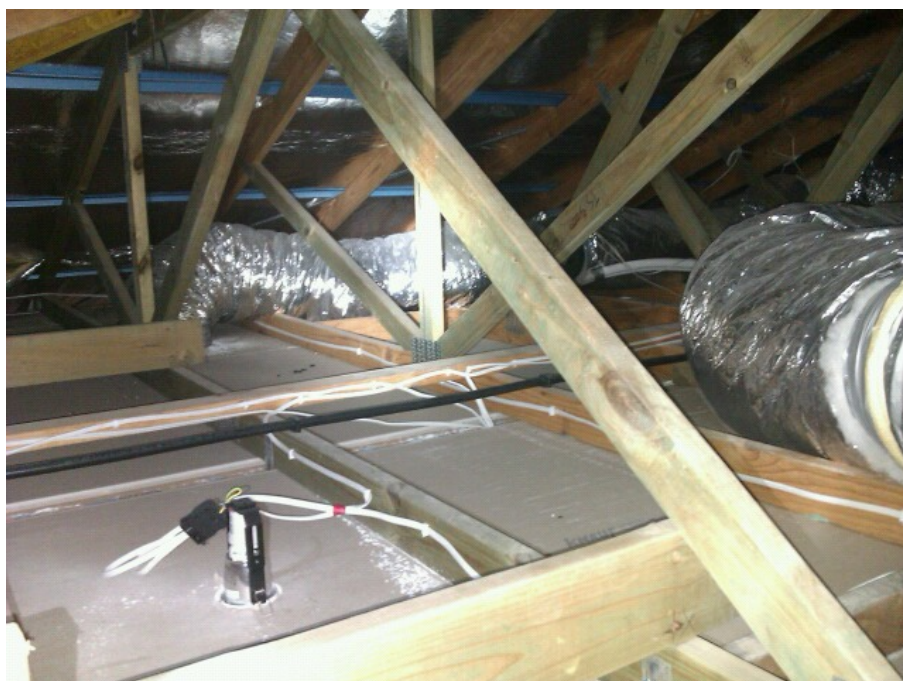
Figure 11 Brisbane house with no ceiling insulation installed
