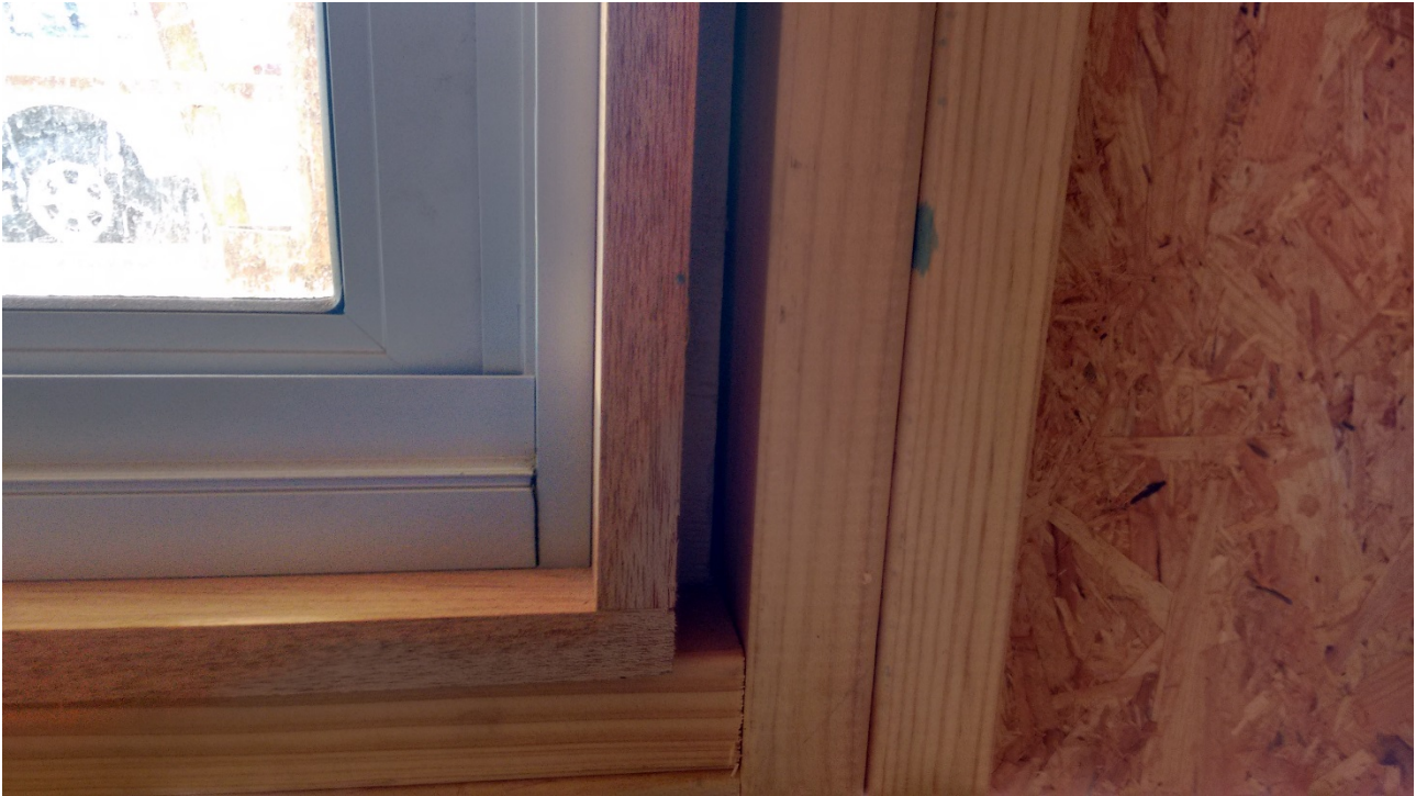
Figure 32 No sealing between window frame and house frame
