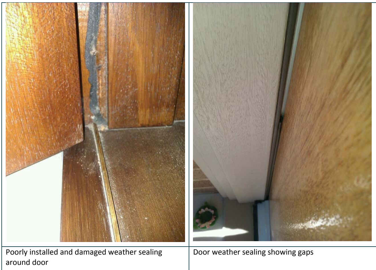
Figure 7 Examples of poor weather sealing on doors
